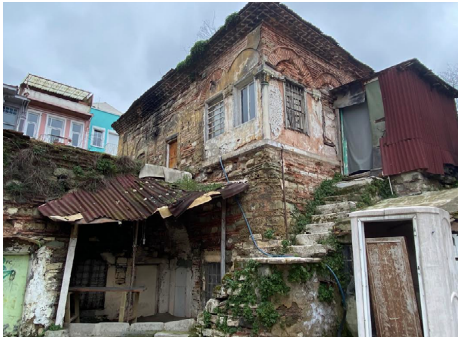
Figure 21: Backside of a masonry wing with portico and staircase, small residence near Sinai Monastery Metochion. Photograph: Firuzan Melike Sümertaş, 2022.
