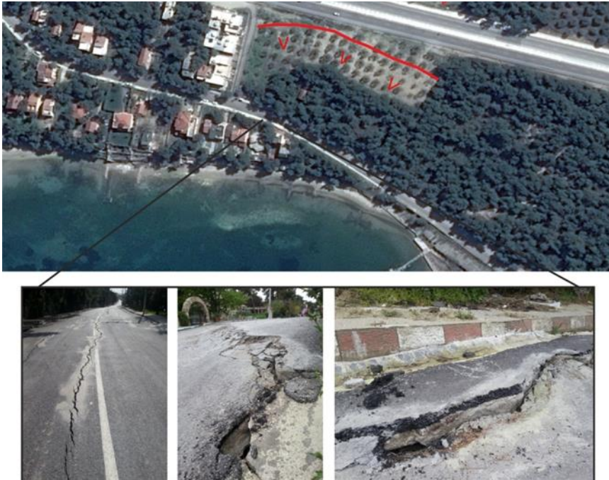
Figure 2. The view of the landslide area on the satellite image and terrestrial photographs of the landslide surface cracks.
