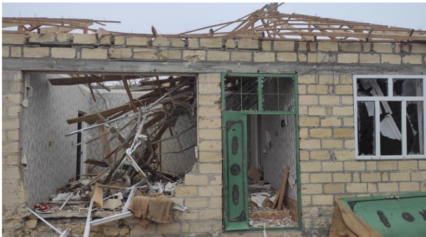
Photograph 3: Destroyed house after the bombing of the village, Garadaghli, Tartar.
