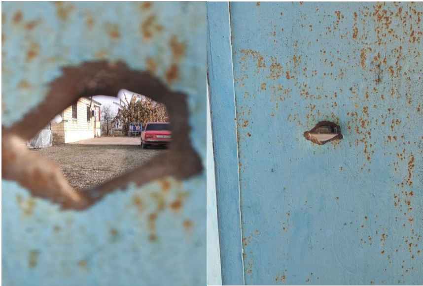
Photograph 1: II Karabakh War traces, bullet hole on the gate, Dordyol, Aghdam
