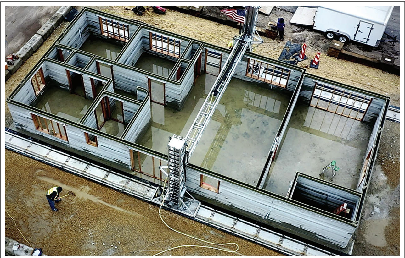
Figure 1. Automated work site with an on-site 3d printer. 3D Autonomous Robotic Construction System (ARCS).
