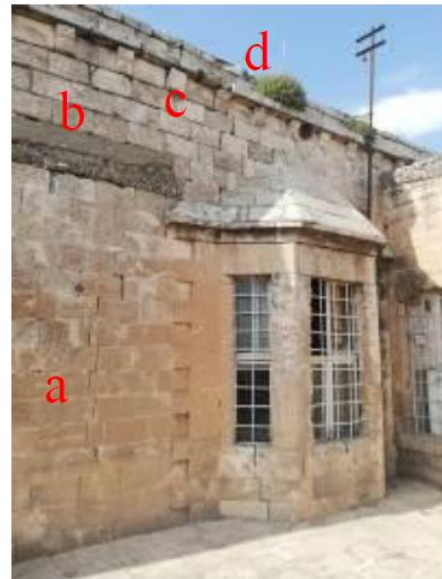
a. Cracks b. Use of cement c. Discharge of jointing d. Plant formation
