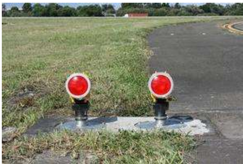
Figure 6. Stop bar Lights [11]
