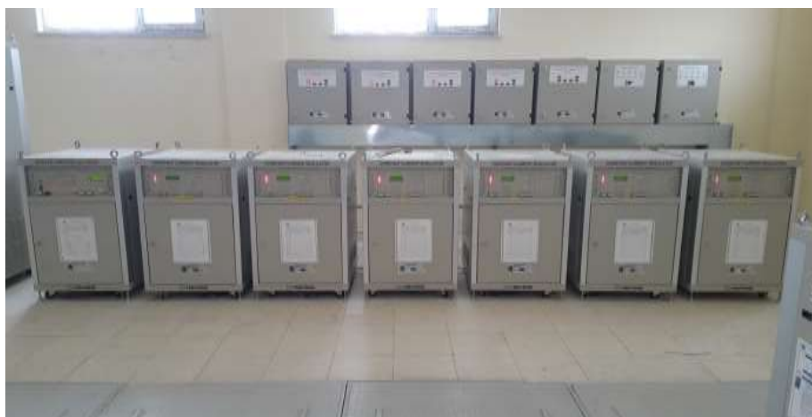
Figure 14. Constant current regulator in transformer building
