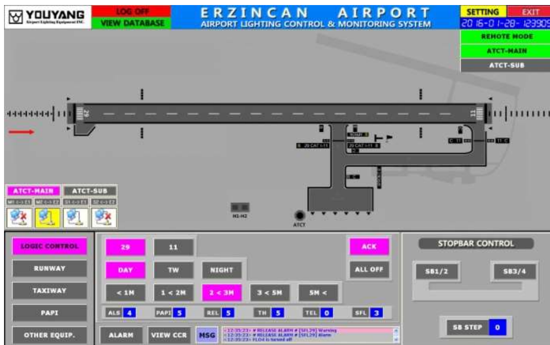
Figure 16. Erzincan airport display of the monitor control lighting equipment except runway
