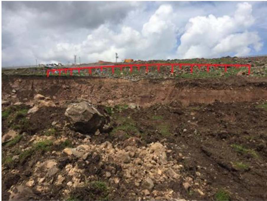
Figure 1. The area where the failure in the study area occurs
