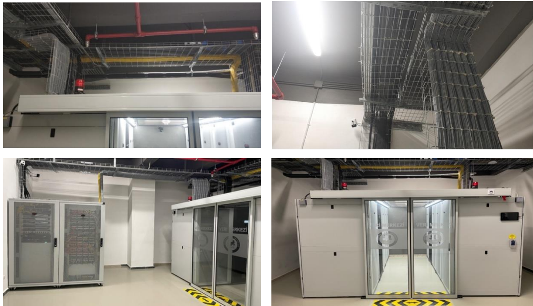
Figure 7. West Campus Data Center
