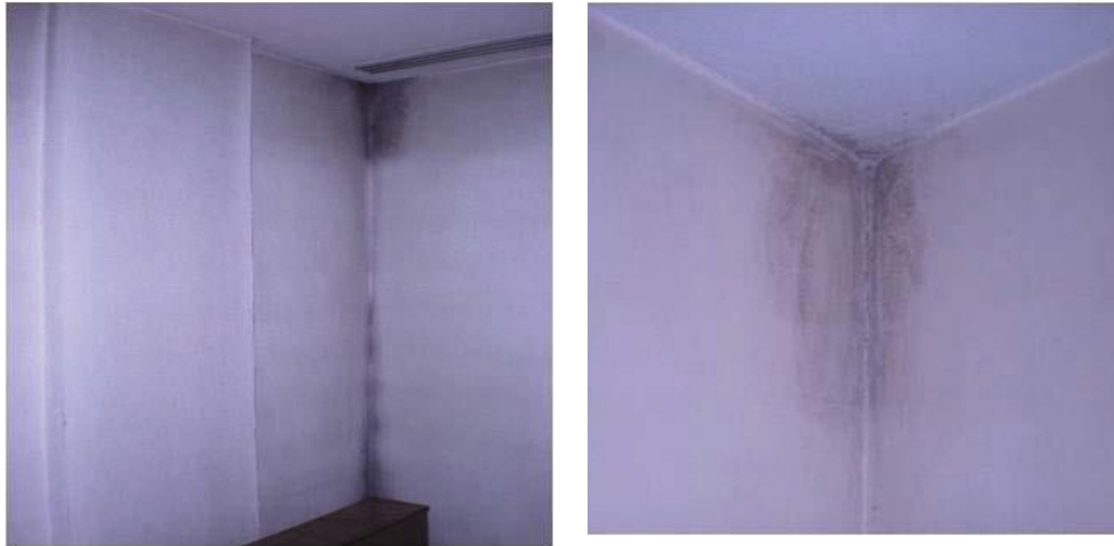
Figure 4. Mold formation in the presence of thermal bridges 29
