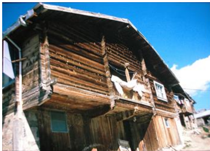
Figure 6. A typical two storey house from Artvin Region (photo belongs to the author).
