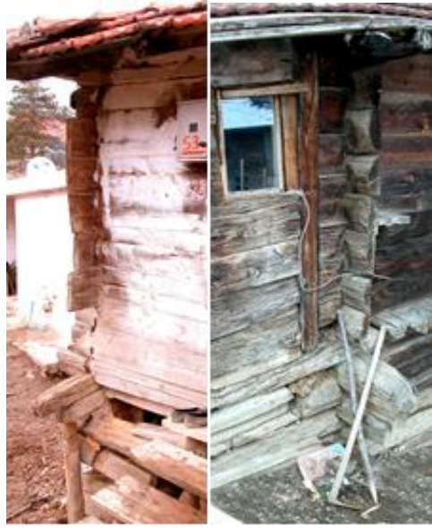
Figure 10, 11. Timber plank connection details from different buildings located high plateaus of Anatolia (photographs belongs to the author).
