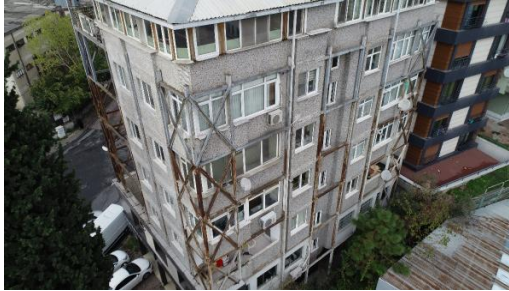
Figure 4. Seismic Bracing Example applied on a residential building at Istanbul, Turkiye (URL-4).
