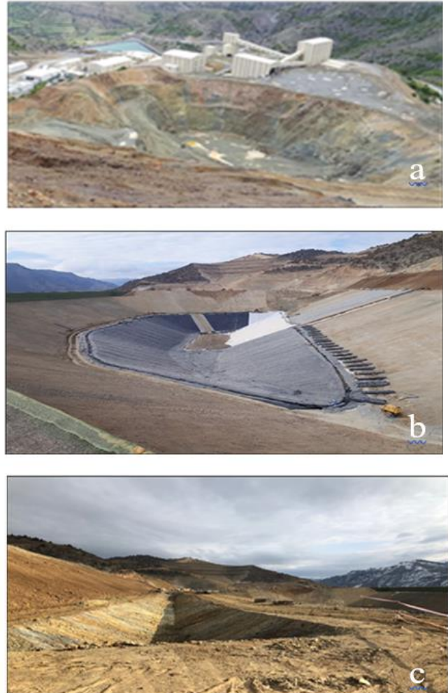
Figure 1 (a) Land view before WST construction (b) geo membrane laying (c) channel construction [23]
