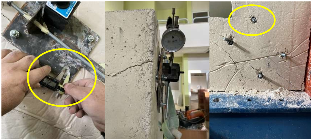
Figure 9. Failure of Strengthening Anchor Bolts at the Junction Area
