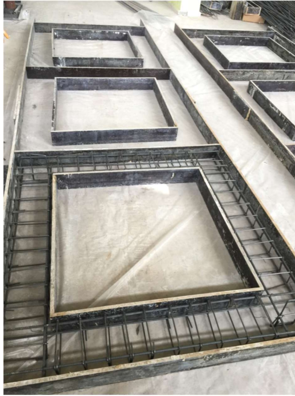
Figure 3. Reinforcement and Formwork Details of Beams and Columns of an RC Frame
