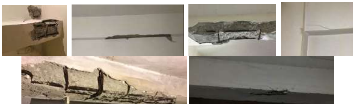
Figure 1. Images of corroded RC beams
