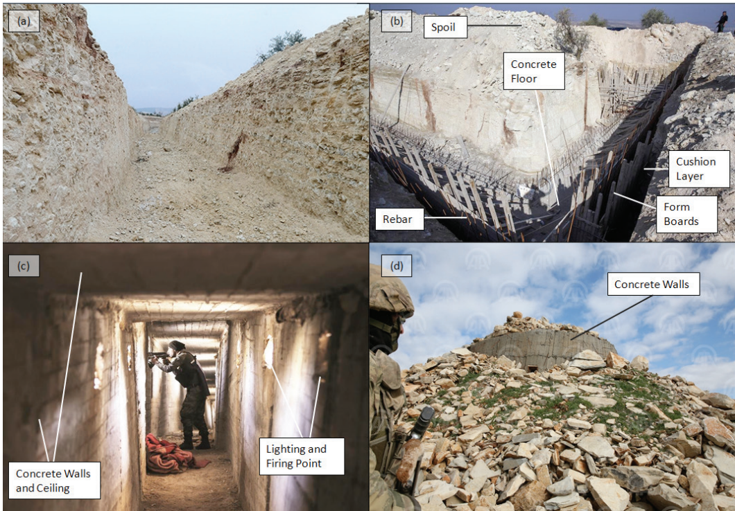
Figure 4. (a). Defensive trench excavated in the mountains around Afrin in horizontally bedded limestone with marls using a mechanical excavator 121 to be used for SDF, YPG and YPJ fighting positions. (b). Construction by SDF, YPG and YPJ of cut-and-cover hardened tunnels at Sirgaya Hill with the concrete and rebar visible along with form boards placed during the concrete pour 122 . (c). SDF, YPG and YPJ CCHT with multiple firing points and dimensions sufficient for a defender to stand 123 . (d). SDF, YPG and YPJ observation point at Mount Bursaya constructed into the mountain slope and camouflaged with limestone blocks to blend into the surrounding terrain 124 .
