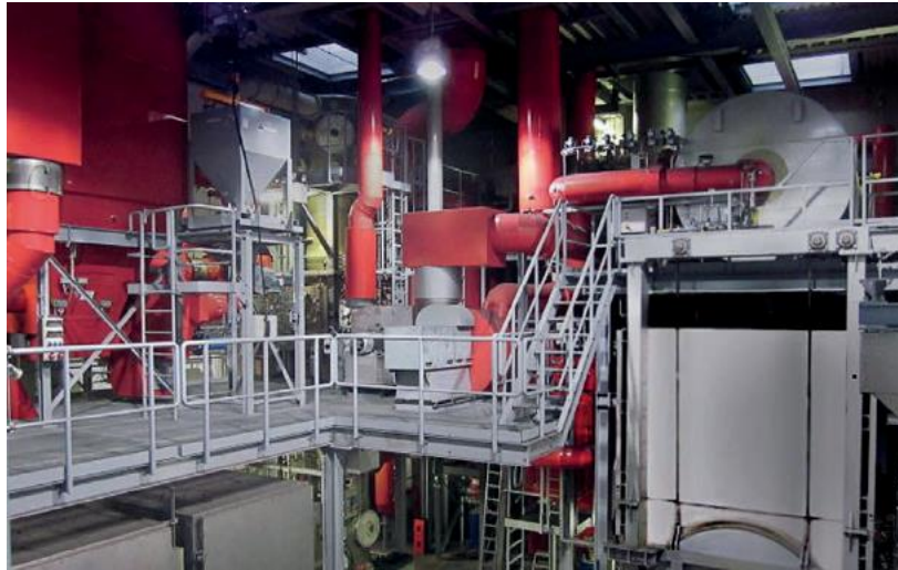
Figure 4: A limestone flue gas desulfurization plant [5].
