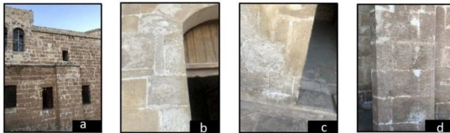
Figure 4. Physical deterioration of Hatuniye Madrasah (Biçen Çelik, 2019)
