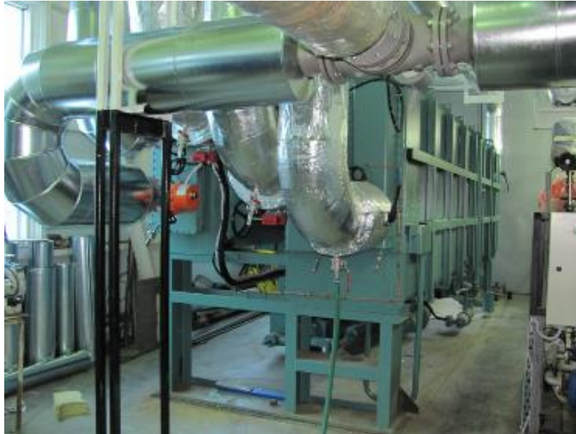
Figure 5. Absorption chiller AR-D500L2 applied in the considered TGP.
