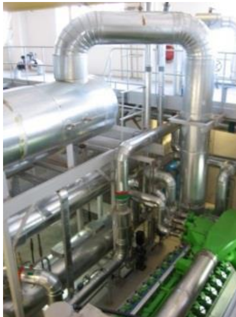
Figure 1. Gas engine cogenerative module JMS GE Jenbacher
