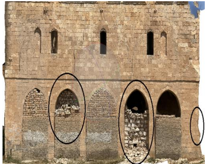
Figure 8. The deformed walls
