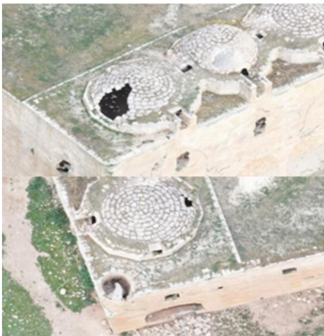
Figure 7. The deformed dome.
