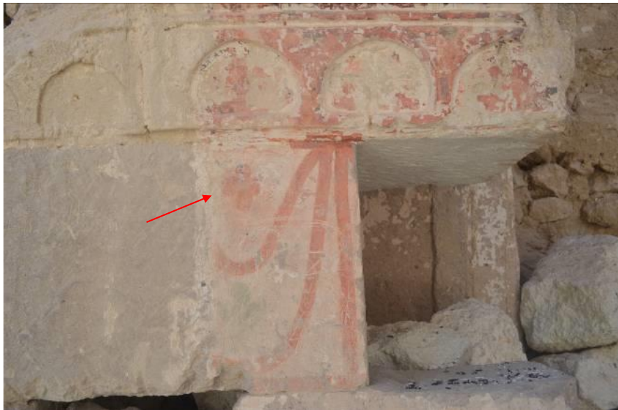
Figure 17: Timos/Tavros Stavros Church, inner surface of the southwest pier of the middle nave; a clover leaf/cross motif on imitation curtain pattern (M. Kaya, 2016)
