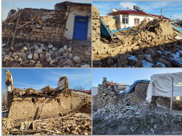
Figure 7. Example of load-bearing wall damages
