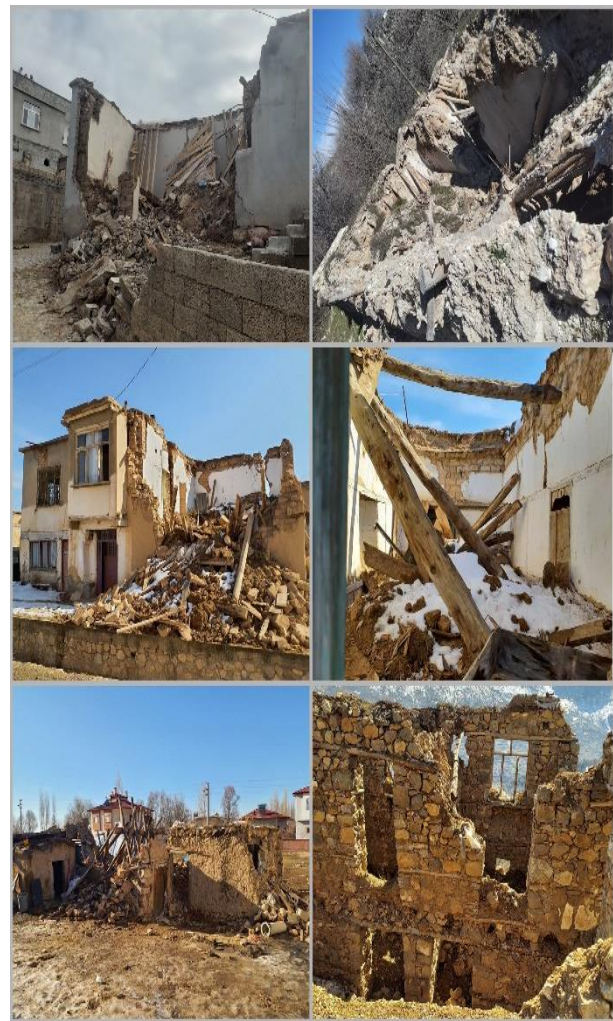
Figure 6. Examples of completely collapsed earthen roofs
