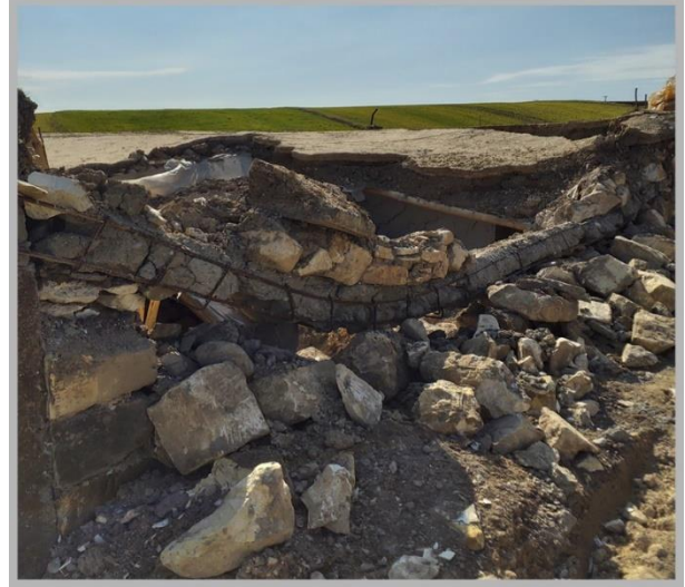
Figure 14. Structural damage despite the use of reinforced concrete bond beams
