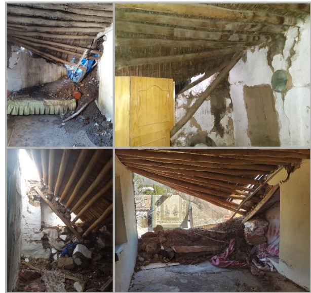
Figure 10. Damages due to insufficient support of wooden beams on heavy earthen roofs
