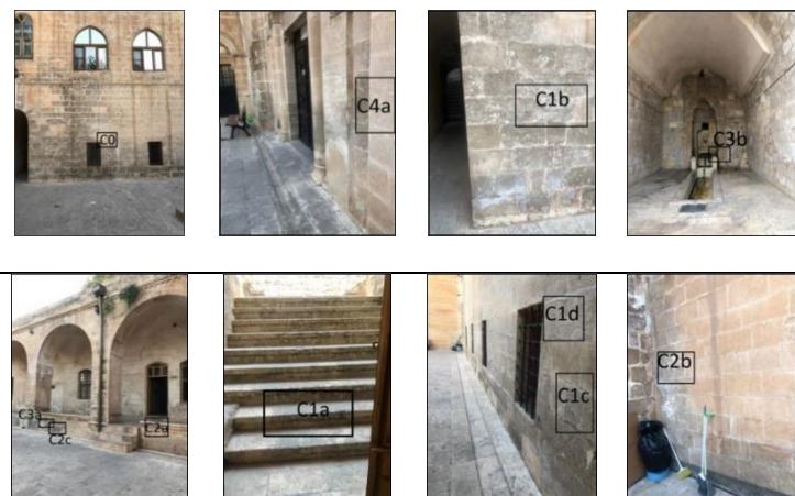
Figure 11. Demonstration of the stones selected for the use of XRF chemical method for the deterioration of Şehidiye Madrasah on the façade
