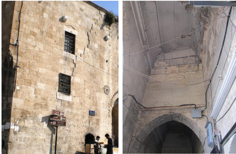
Figure 32. The Structural Problems Observed in the Khan's Northwestern Section (Kasmo, 2010)
