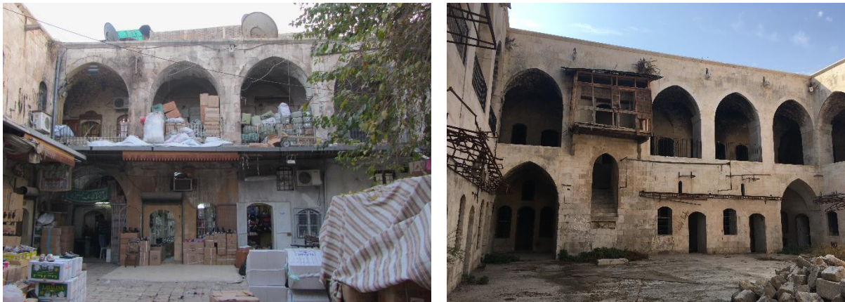
Figure 11. General Views of the Courtyards of Khan al-Absi, on the left, (Kasmo, 2011) and Khan al-Haj Musa, on the right, (Grandin, 2020©) showing the absence of preceding porticoes on ground floors.
