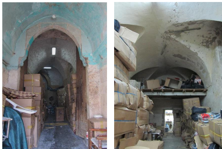
Figure 12. The Entrance, on the left, and a General View, on the right, of the Khan's Stable (Kasmo, 2010)
