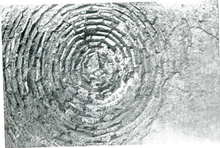
Res. 30 — Kuzey galeriyi örten kubbecikler. Fig. 30 — One of the small domes above the Northern gallery.
