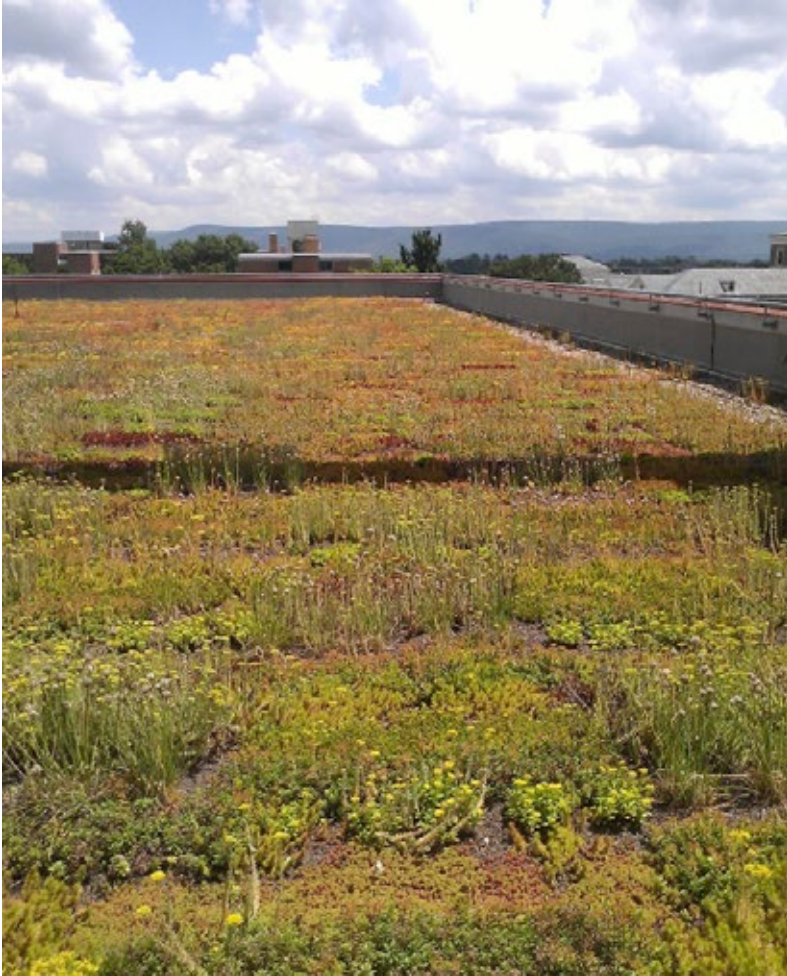
Image: Green roof on Penn State University (self-credit)
