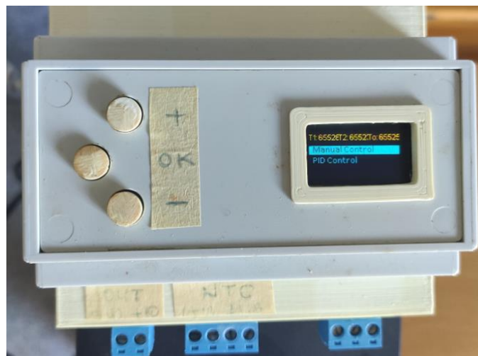
Figure 4. PID Control device
