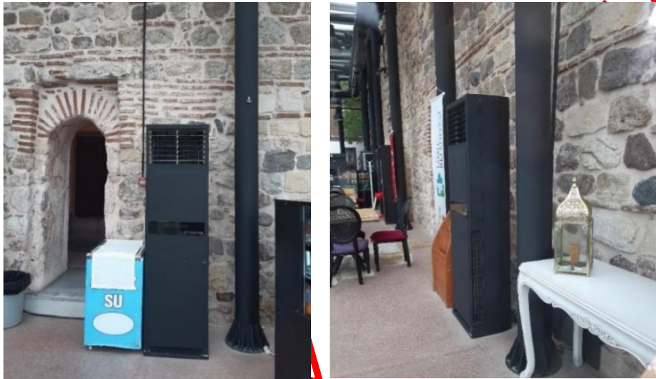
Figure 7. HVAC systems used in the restaurant of Süleyman Pasha Hamam (Personal Archive)
