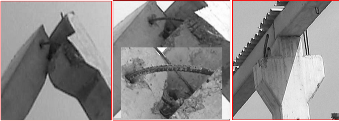
Figure 6. Failure of connection
