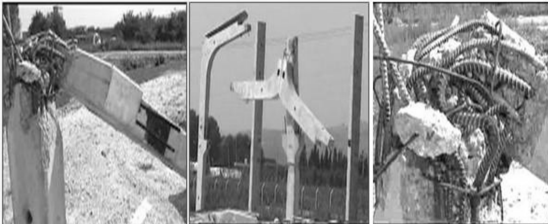
Figure 18. Two spanned column damage
