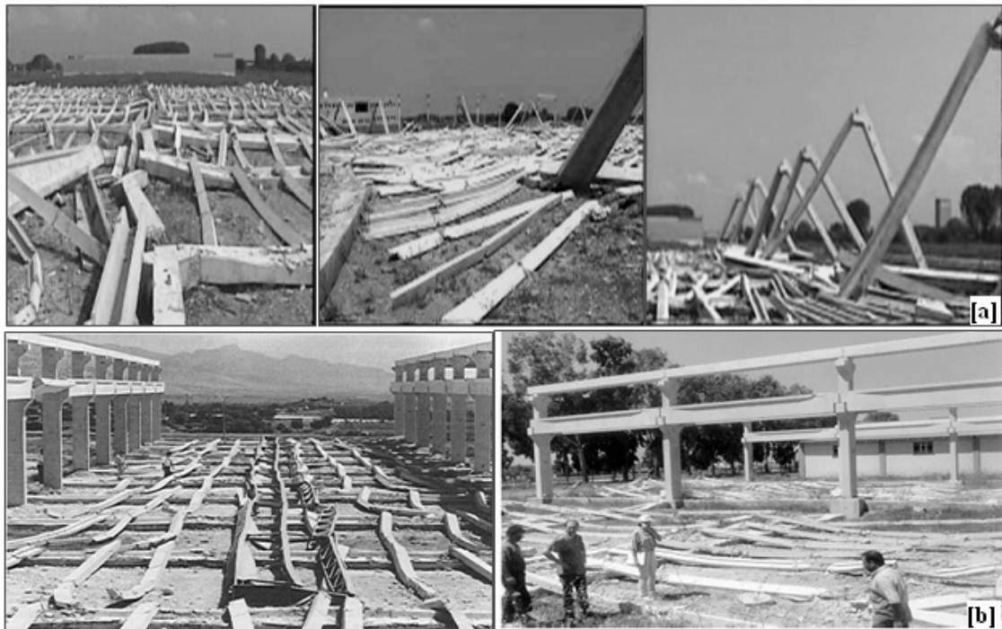
Figure 5. Prefabricated Structure damage a-Ceyhan b-Kocaeli earthquake
