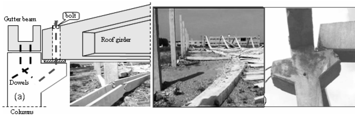
Figure 16. Gutter beam (a) connection section (b) damage
