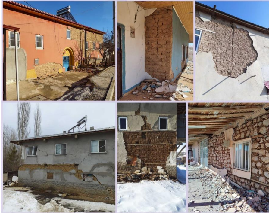
Figure 9. Falling of exterior materials
