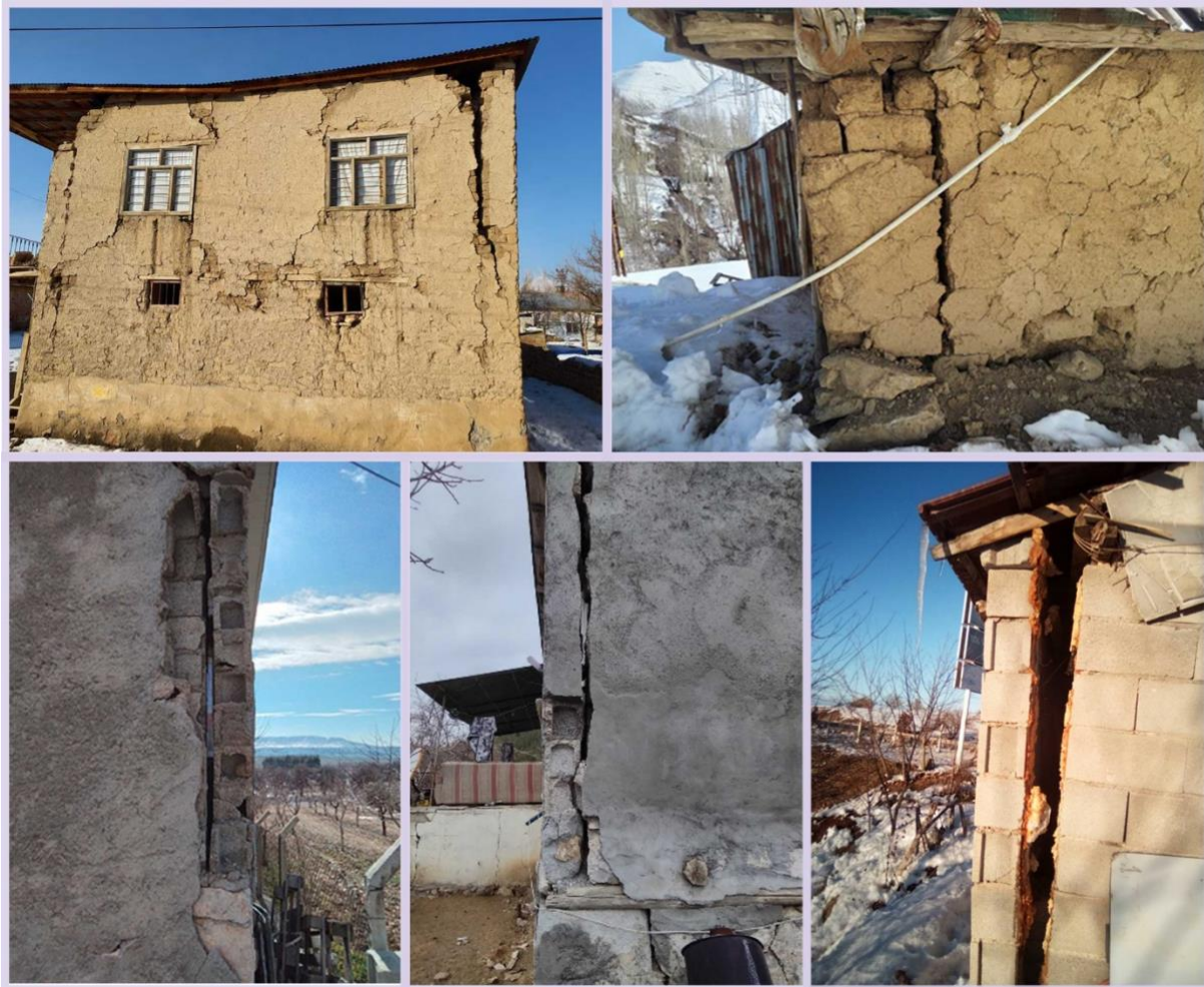
Figure 6. Wall separation at corners of the structures
