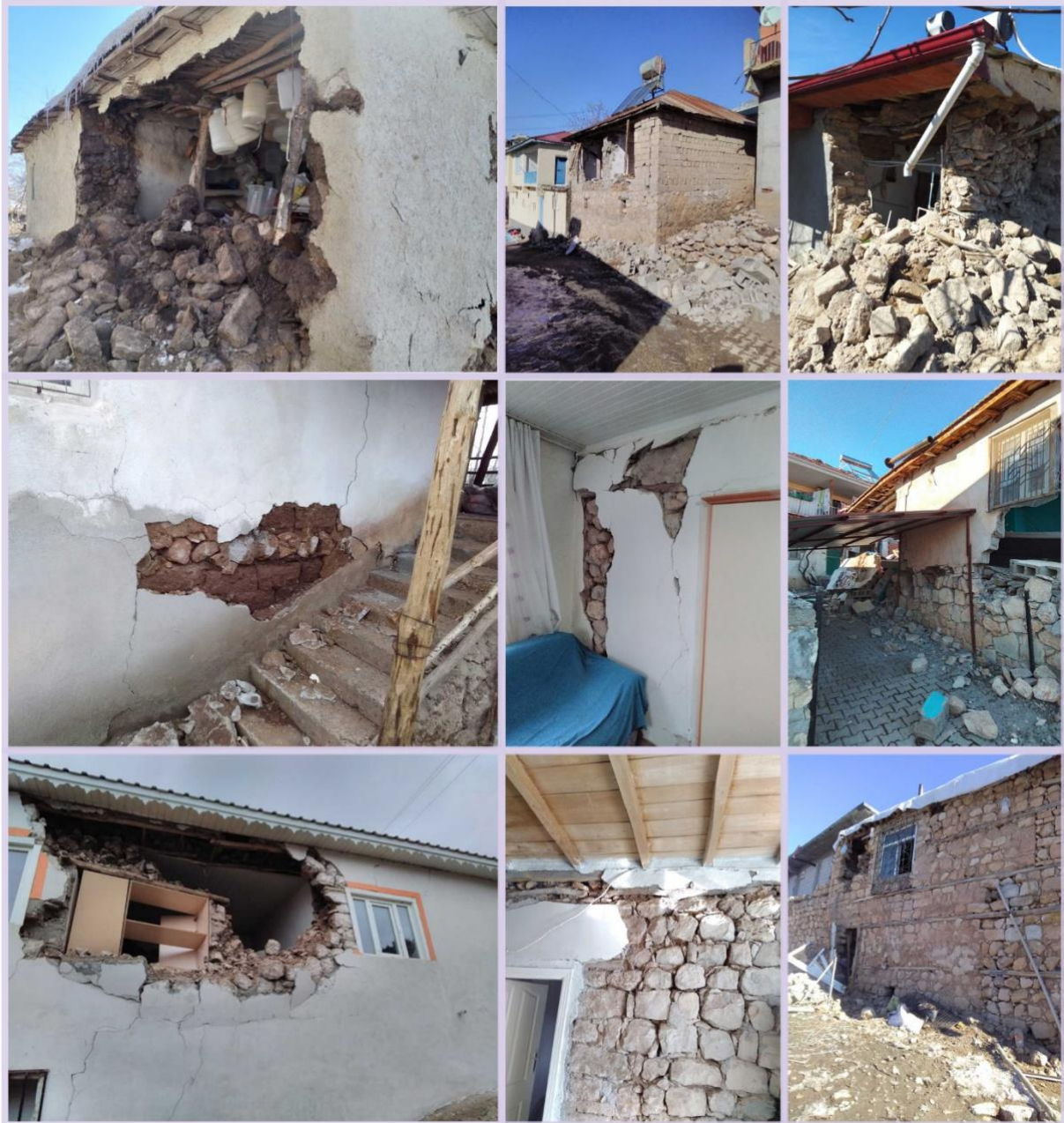
Figure 12. Examples of wall damage caused by various reasons
