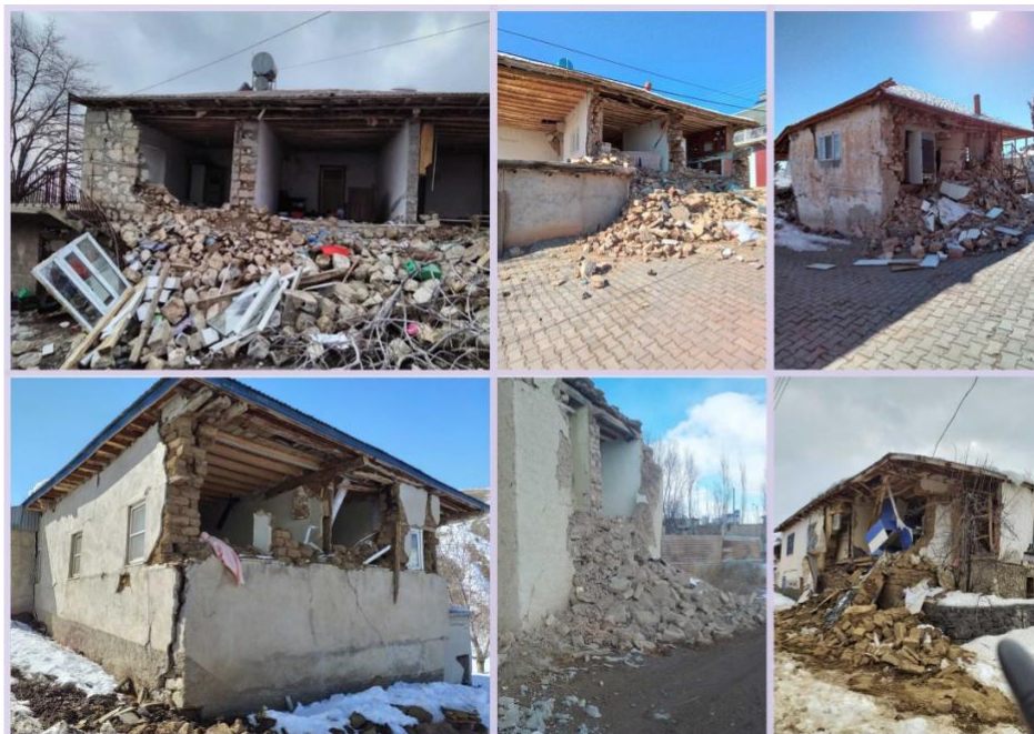
Figure 10. Example of out-of-plane movement on load-bearing walls
