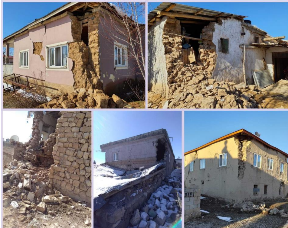
Figure 8. Examples of out-of-plane wall corner damage
