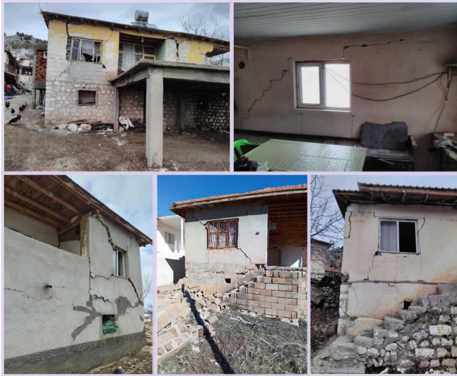
Figure 7. Damages at window corners
