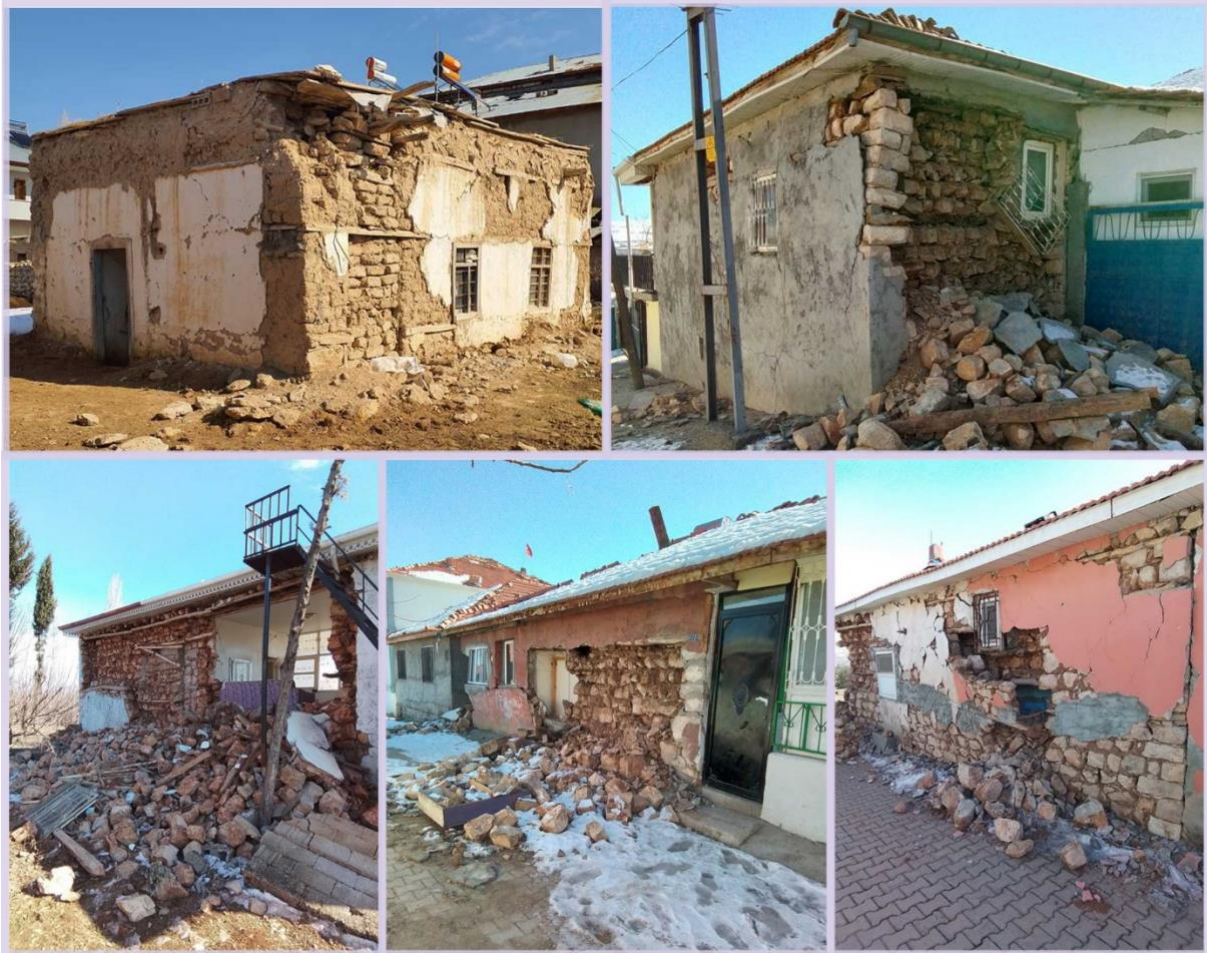
Figure 11. Examples of damage caused by inadequate connections between layers
