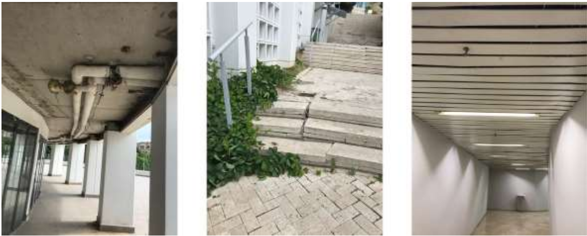
Figure 11. Some images showing the problems in need of repair and maintenance (Nalçacıoğlu, 2022)
