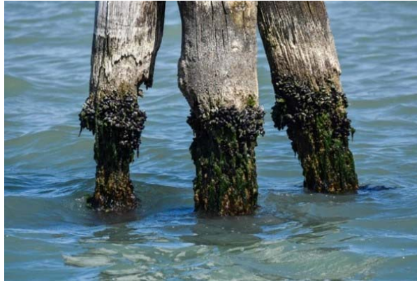
Figure 12. Damage on wood in marine (Wooden bricole, wooden mooring poles in the water, Venice, Italy, 2019 Free Photo, 2024).
