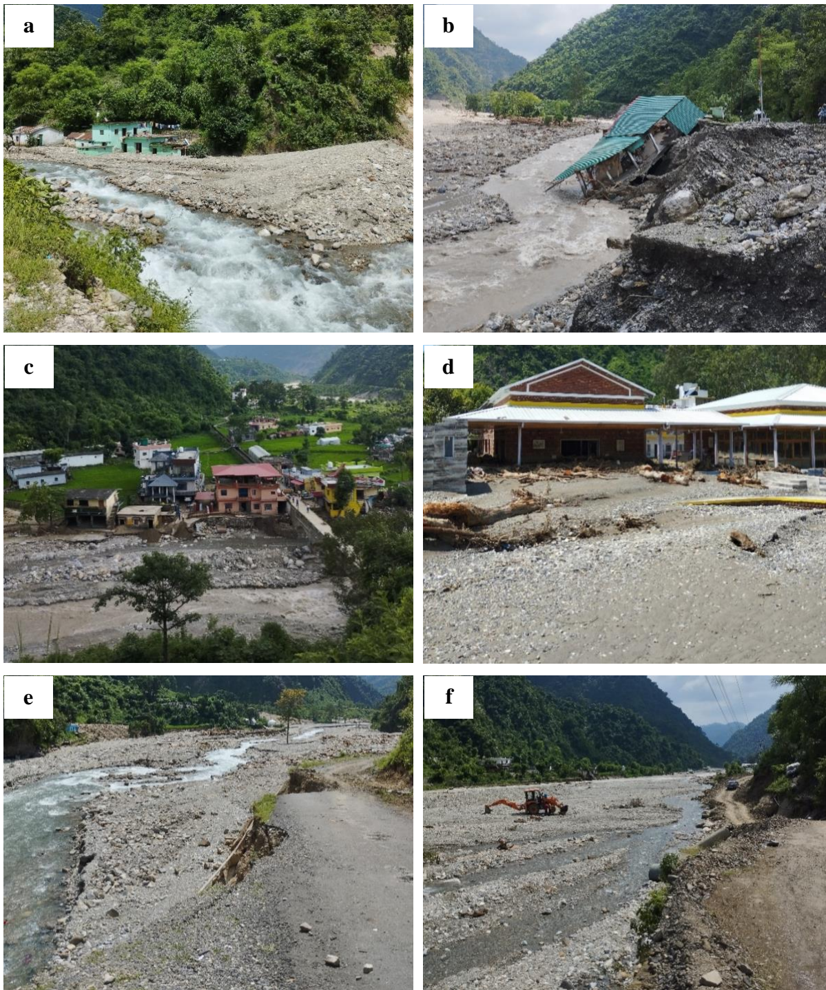
Figure 4. Flash flood damages in both the banks of Bandal Nadi ; (a) Damage to habitation of Dhantu Sera on the left bank, (b) damage to a building located East of Bouta at right bank, (c) Houses damaged at village Kumalda on the left bank, (d) damage to Four Banyans Spirit & Nature Resort downstream of the confluence of Bandal Nadi & Song Nadi , (e) washed away road on the right bank between Dhantu Sera and Bhaishwar villages, and (f) wiped out road between Sarkhet and Bhaishwar area on the right bank
