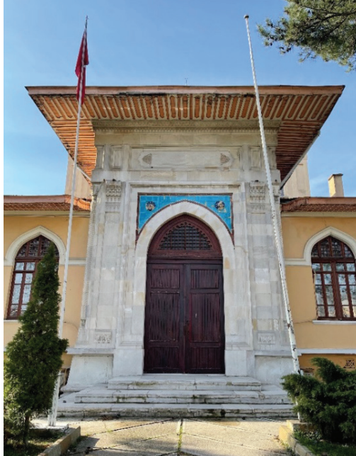
G. 4: Edirne Union and Progress Club Building, Crown Door View, (A. Balcı, 2022)
