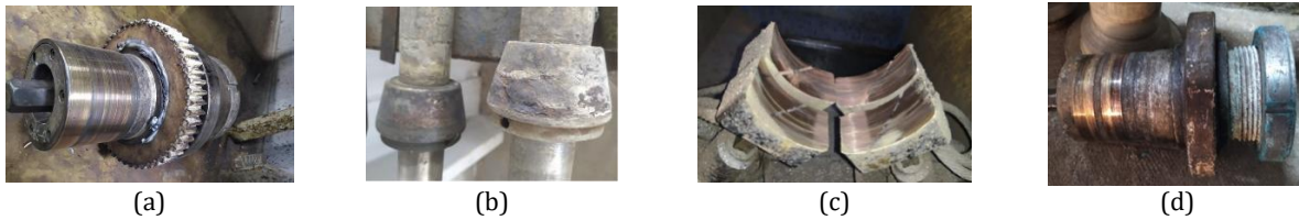
Figure 8. Deteriorations in Plating Bath Because of Heating Caused By Current Imbalance: A) Melted Adapter Gear, B) Taper Distortion, C) Adapter and D) Coals.
