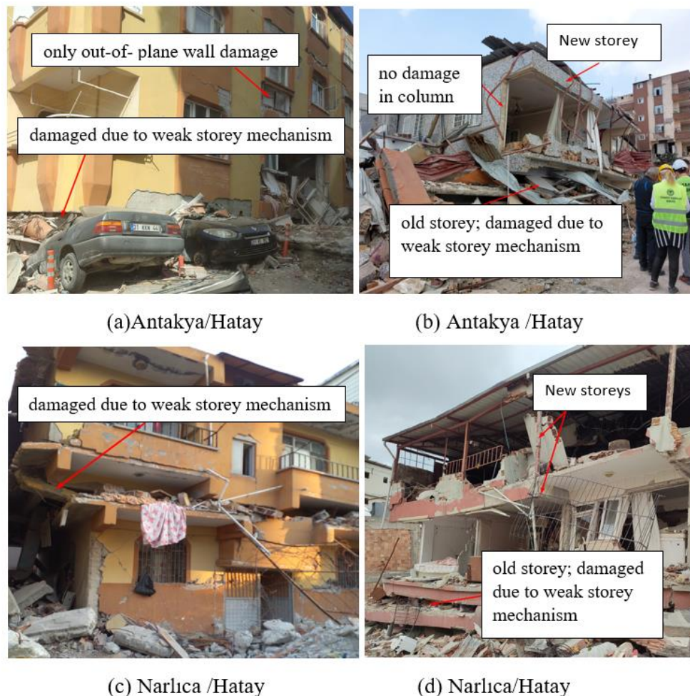
Figure 16. Observed structural damages in the earthquake region. RC building damage related to the weak storey mechanism. (a) Building, located in Antakya/Hatay, collapsed on the ground floor, while the upper floors had only wall damage; (b) Building, located in Antakya/Hatay, collapsed on the ground floor, yet the upper floor had no damage in beam-column joints; (c) Building, located in Narlıca/Hatay, collapsed on the second floor; and (d) Building, located in Narlıca/Hatay, collapsed on the first and second floors.
