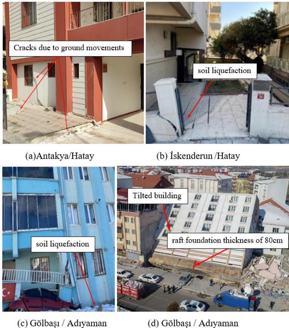
Figure 17. The foundation failure in (a) Antakya-Hatay, (b) İskenderun-Hatay (Cetin et al., 2023)), (c) Gölbaşı-Adıyaman (Cetin et al., 2023)) and (d) Gölbaşı-Adıyaman (adapted from (Bilgin, 2023; Cetin et al., 2023)).
