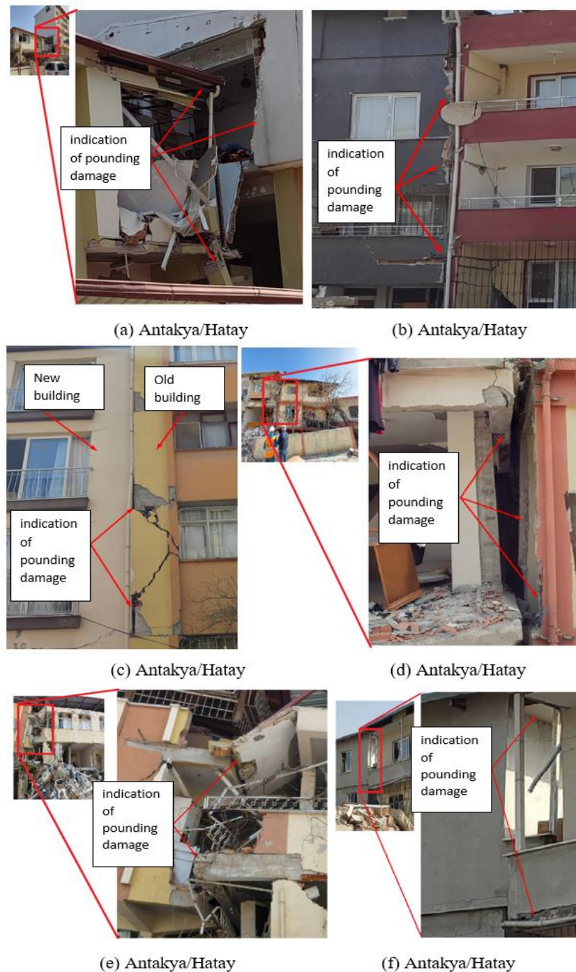
Figure 10. Observed structural damages in Antakya/Hatay. Damages due to adjacent buildings' lateral displacement. (a) A 7-story building collided with a 2-story building. (b and c) 4-story new and old buildings collided with each other. (d, e and f) 2-story old buildings collided with each other.
