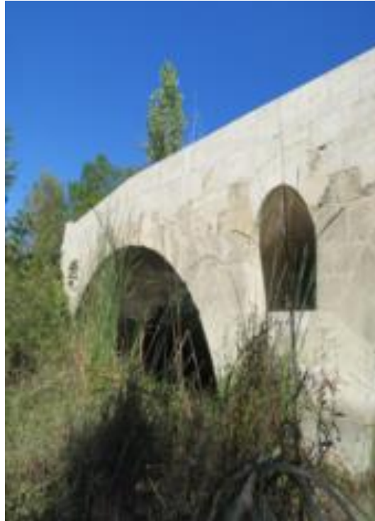
Figure 10. Detail of the First Arch and the Discharging Arch (Photo: İ. Göçmen)
