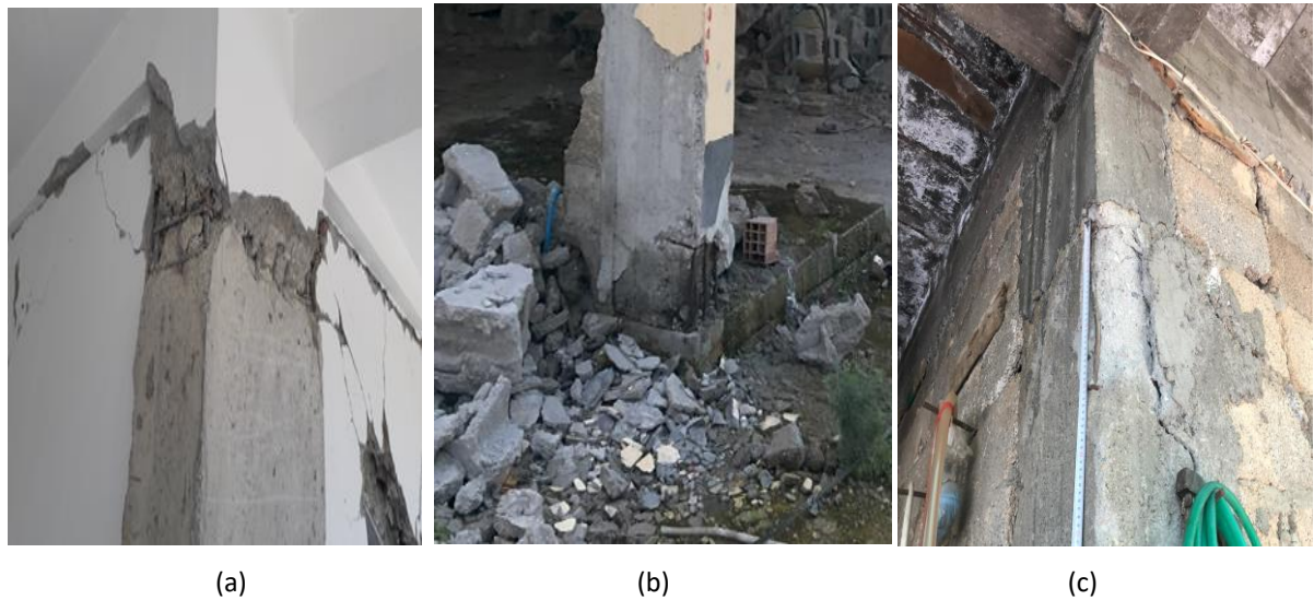
Figure 5. Structural damage types (a), (b) core crushing, shell crushing, shell crushing, reinforcement buckling, (c) insufficient transverse reinforcement - Malatya; (Karataş, 2023)
