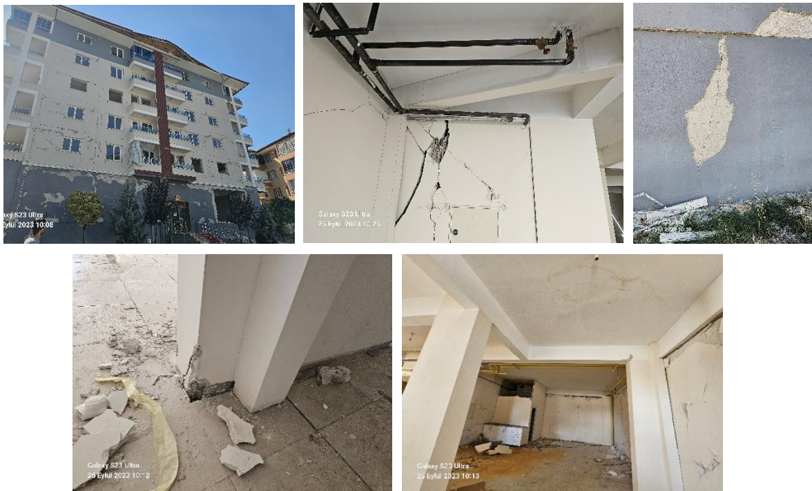
Figure 10. Soft Floor Effect Damage - Malatya (Karataş, 2023)
