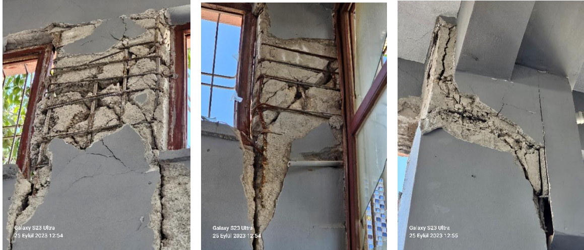
Figure 7. Damages resulting from manufacturing errors - Malatya (Karataş, 2023)
