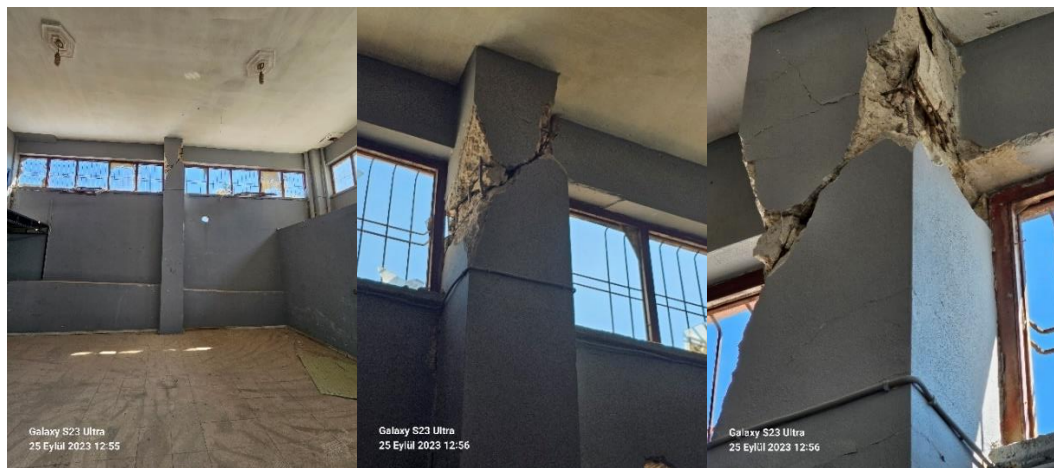
Figure 8. Short colon effect damages – Malatya (Karataş, 2023)
