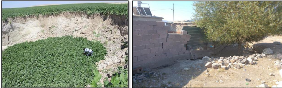
(f) A sinkhole formed in the beet field on 23 Aug 2016
