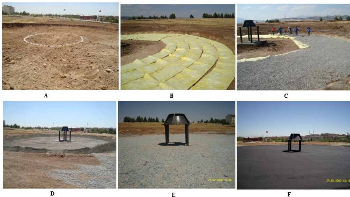
Figure 4. Pictures showing the construction steps of ground of solar tower system A ground floor, B Aluminum folio with glass wool, C Gravel laying, D Sand, E Glass laying, F Asphalt paved.
