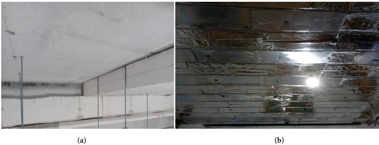
Figure 7. Thermal insulation layers of the ceiling. (a): Fixing two-layer polystyrene of thickness 4 cm of each layer below the ceiling. (b): Attachment of the last 4 cm polystyrene layer with 1 cm aluminum layer.
