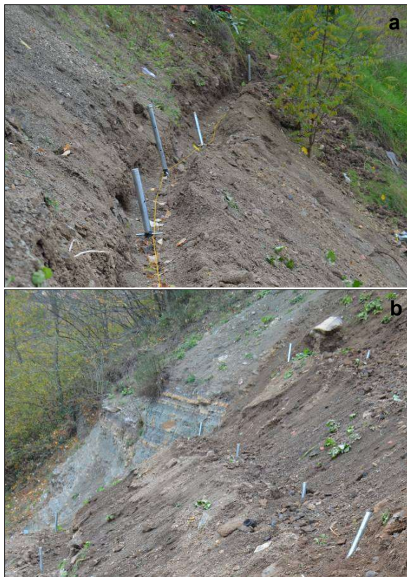
Fig. 9. a) A close up view (during the installation phase) and b) A general view of the cable fixing points (upon installation) within the landslide footprint area.
