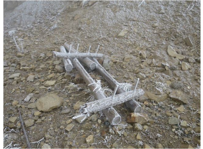
Figure 7. Damaged and Fallen Parts of Wooden Snow Supporting Structures (2014)
