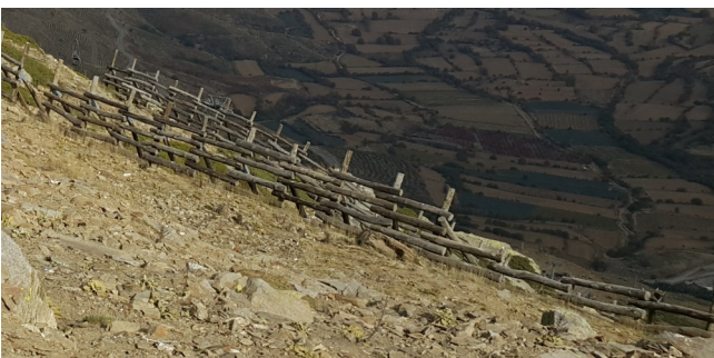
Figure 6. Wooden Snow Bridges and Their Condition After Avalanche (2015) –G. Arslan
