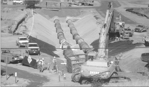
Fig 15. Fault Crossing Design of 66-inch Pipeline San Francisco Hetchy Hetchy Water System in special trench [10]
