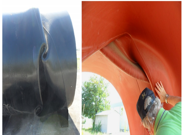
Figure 6. Failure of ductile welded steel water pipe due to excessive compression strain (abrupt PGD) (fault crossing) in Kullar [5, 12]
