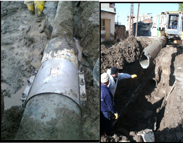
Fig 4. Damaged and repaired joints of segmented A/C water pipes (2011, Van earthquake) [2]
