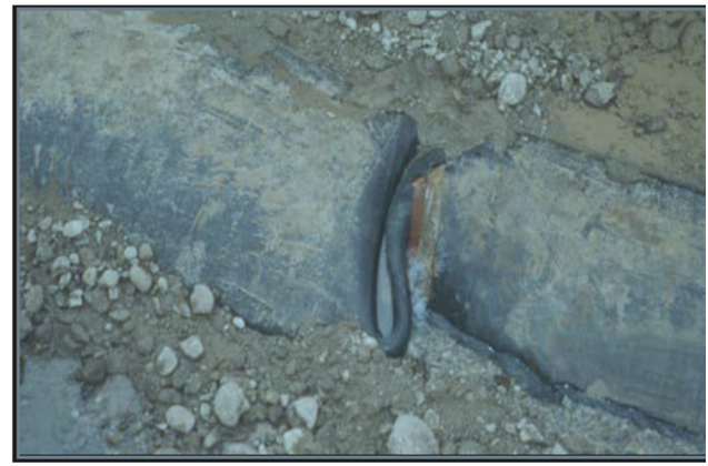
Fig 5. Wrinkling of the main water transmission pipe due to strike slip fault offset (abrupt PGD) in the 1999 Kocaeli earthquake [7], [12]
