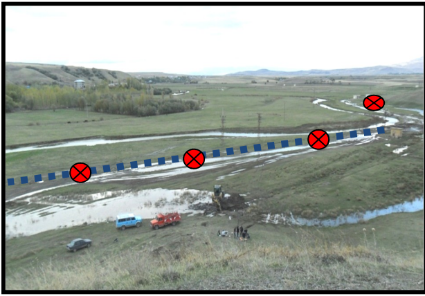
Fig 3. Damage locations of water transmission pipe due to liquefaction induced lateral spreading and settlement in 2011 Van, Turkey earthquake (spatially varying PGD hazard)
