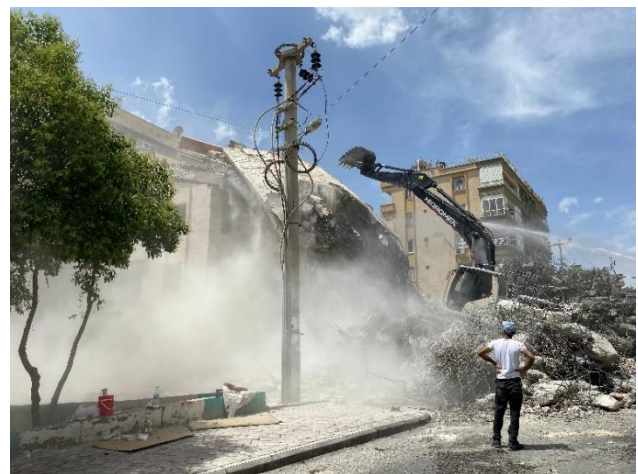
Figure 1. Demolition of a building generating significant PM emissions, illustrating the environmental impact of demolition activities on air quality (Şanlıurfa 2024)
