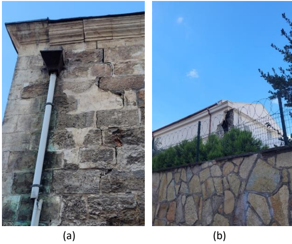
Figure 9. (a) Proper connection of quoin stones, Karagöz Mosque, Gaziantep. (b) Insufficient connection of quoin stones, St. Nicholas Orthodox Church of Iskenderun, Hatay.
