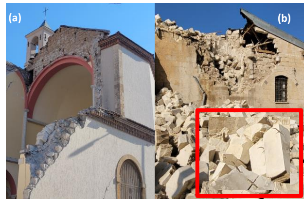
Figure 7. (a) Rubble stone masonry disintegration due to poor quality of materials, (b) cut stone disintegration due to opened metal connector equipment in between.
