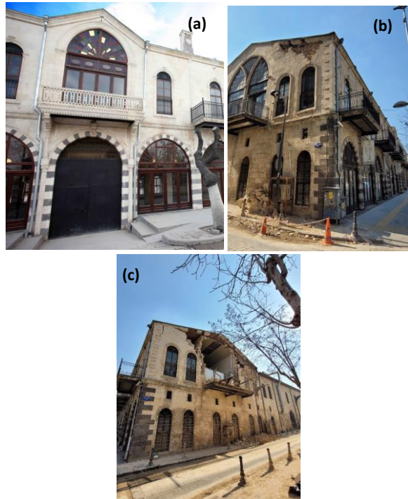
Figure 12. Bayazhan in Gaziantep, (a) Bayazhan before Kahramanmaraş earthquakes (Photo Credit: Gaziantep Provincial Directorate of Culture and Tourism). (b) Damage at the walls of the east side of Bayazhan. (c) Damage at walls the west side of Bayazhan.
