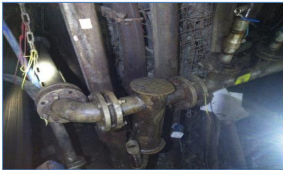
Şekil 10. Metan drenaj boru şebekesinden su tahliye sistemi. Figure 10. Water evacuation system from methane drainage pipe network.
