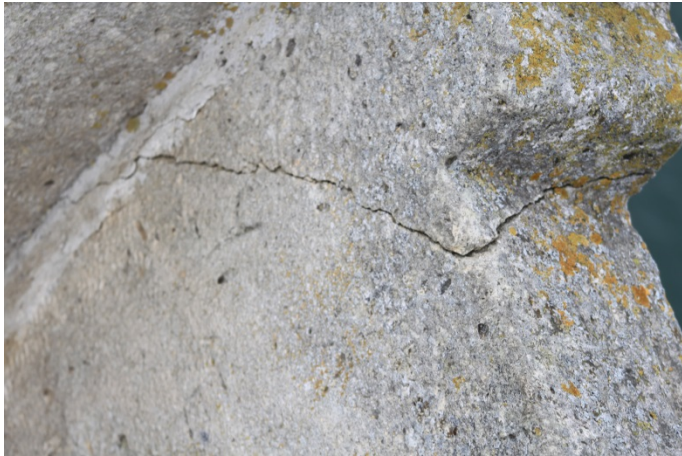
Photo: 6. Buyukcekmece Bridge (Cracks and Fractures)
