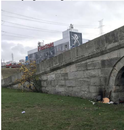
Photo: 8. Kapuagasi Bridge (Surface Accumulation)
