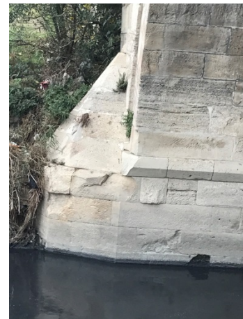
Photo: 10. Kapuagasi Bridge (Fragmentation)
