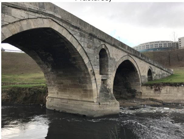
Photo: 7. Kapuagasi Bridge (Surface Accumulation)
