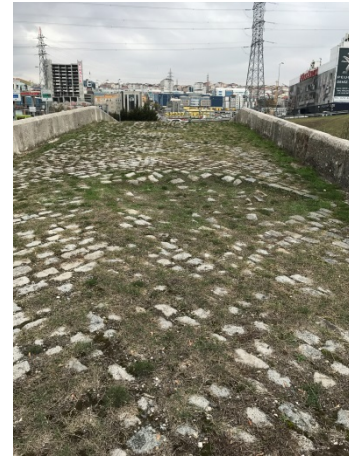
Photo: 9. Kapuagasi Bridge (Damages)
