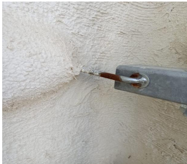
Figure 3. Corrosion at the joint between the GFRC panel and steel frame
