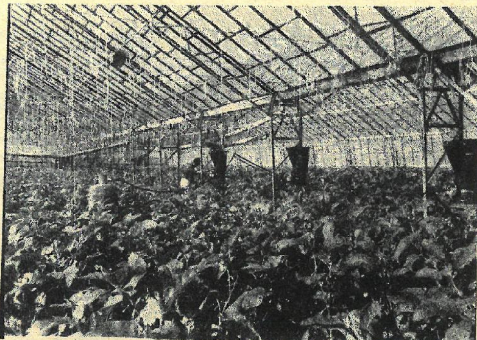
Figure 10. LPG tubes inside the greenhouse
