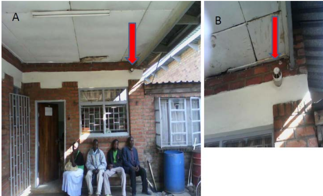
Figure 4. Improperly placed exhaust ducts at Limbe Health Centre. Exhaust duct facing the patients' waiting area (courtesy of Jonathan Majamanda and Philmon Ndhlovu)
